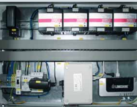
Data concentrators using advanced CAN bus technology can do more than control up to 240 multi-color sensors
